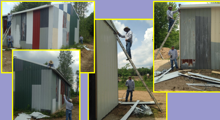
Art, Hipolito, Natalio & Sebastian installed soffit, fascia and doors at the Bowers pole barn. Mike Holton has painted the pole barn one color & looks very nice.
