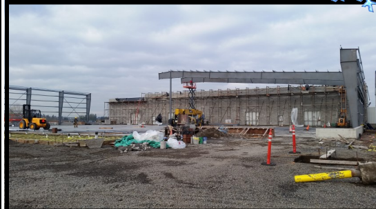
First pair of roof trusses going up. The block wall in the background is almost complete.
